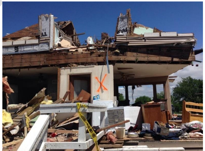
2014 Wessington Springs Tornado Damage (Photo from SDPB website)
